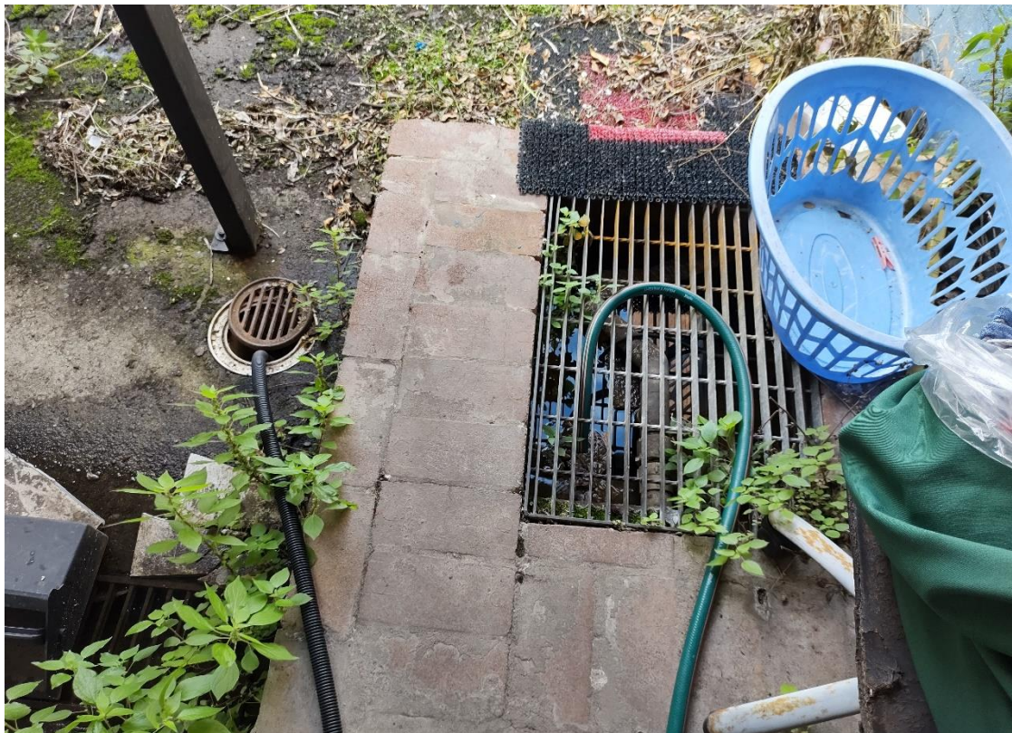
Photo 6: Rear of drycleaner, stormwater and sewer network (potential release point for PCE)
